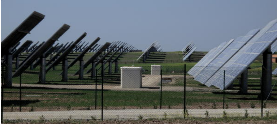
Figure 5: The two white boxes in the centre of the picture are inverter units that receive DC power from the panel assemblies and output AC power to the plant substation.
