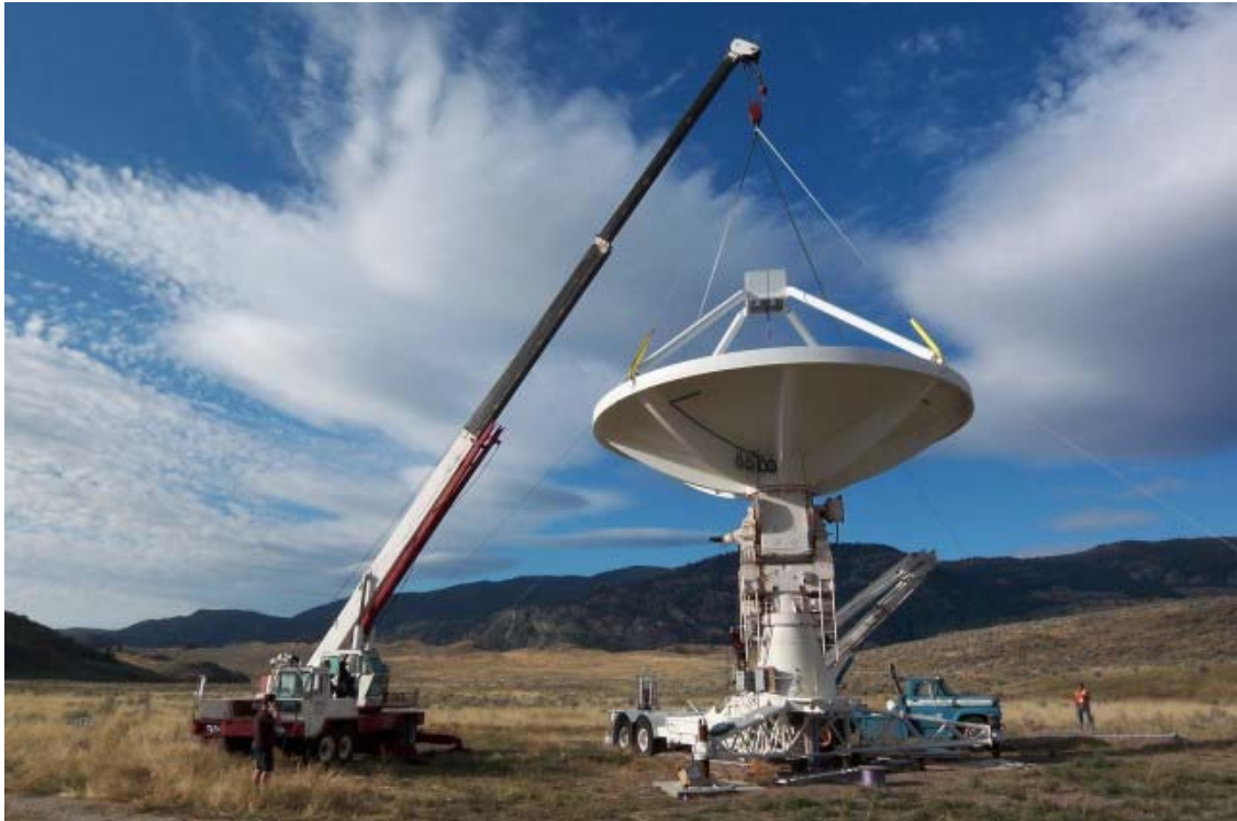
Figure 2. CART Mk2 Reflector being lifted into place September 12 th . The housing for the PHAD array is visible at the focus.
